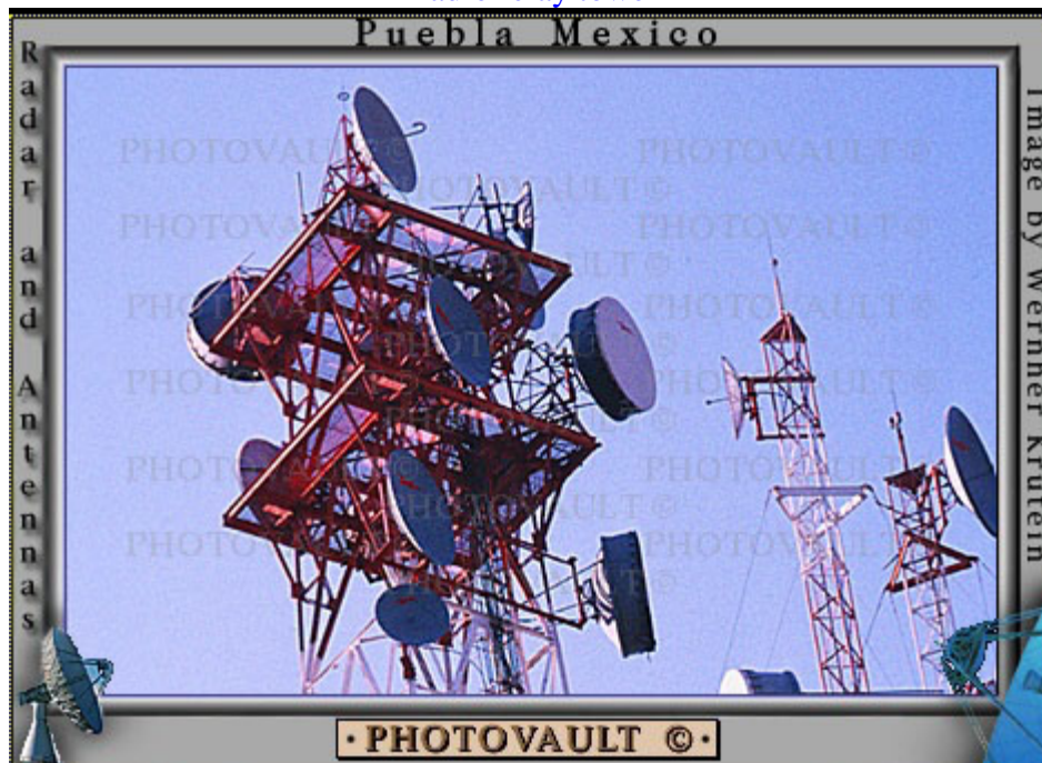
Radio relay tower
