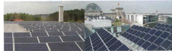
Panels mounted on a flat roof
